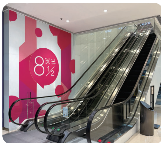
Service-on-Demand Escalator at 8½ Retail Arcade
