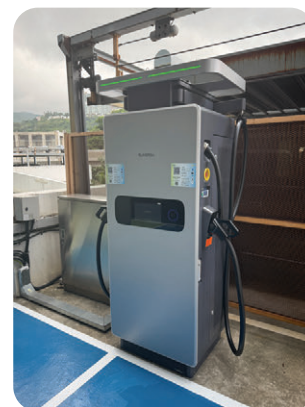
EV Charging Stations at CDW Building Carpark
